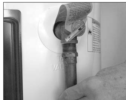
Figure 16 - The T&P Relief Valve discharge pipe must be installed properly and piped to an adequate drain.
